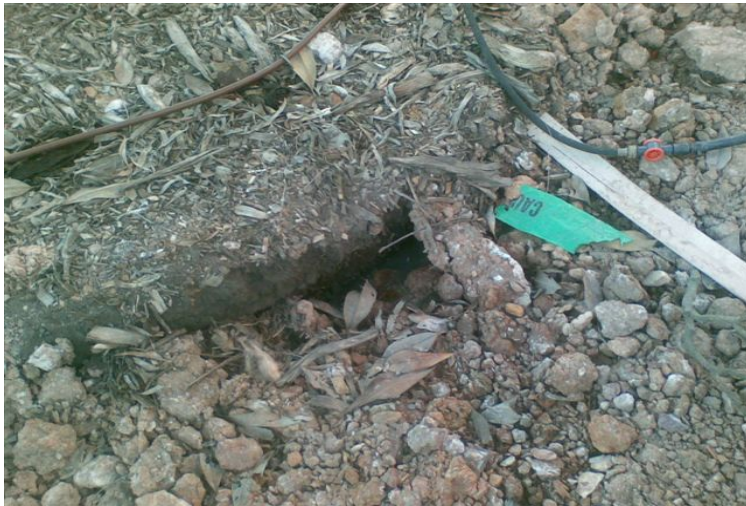
Soil interface issues, water pooling between interface
